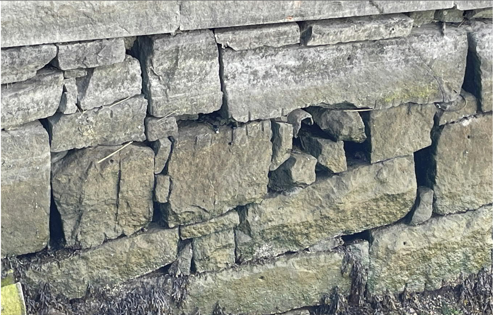
B – View of seawall, note some loss of blocks and opening of joints. Moderate portions have this level of damage.
