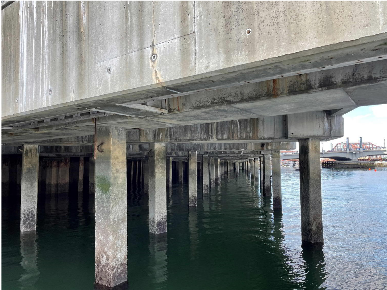
C – Detail view of crack in concrete deck structure and condition of piles.
