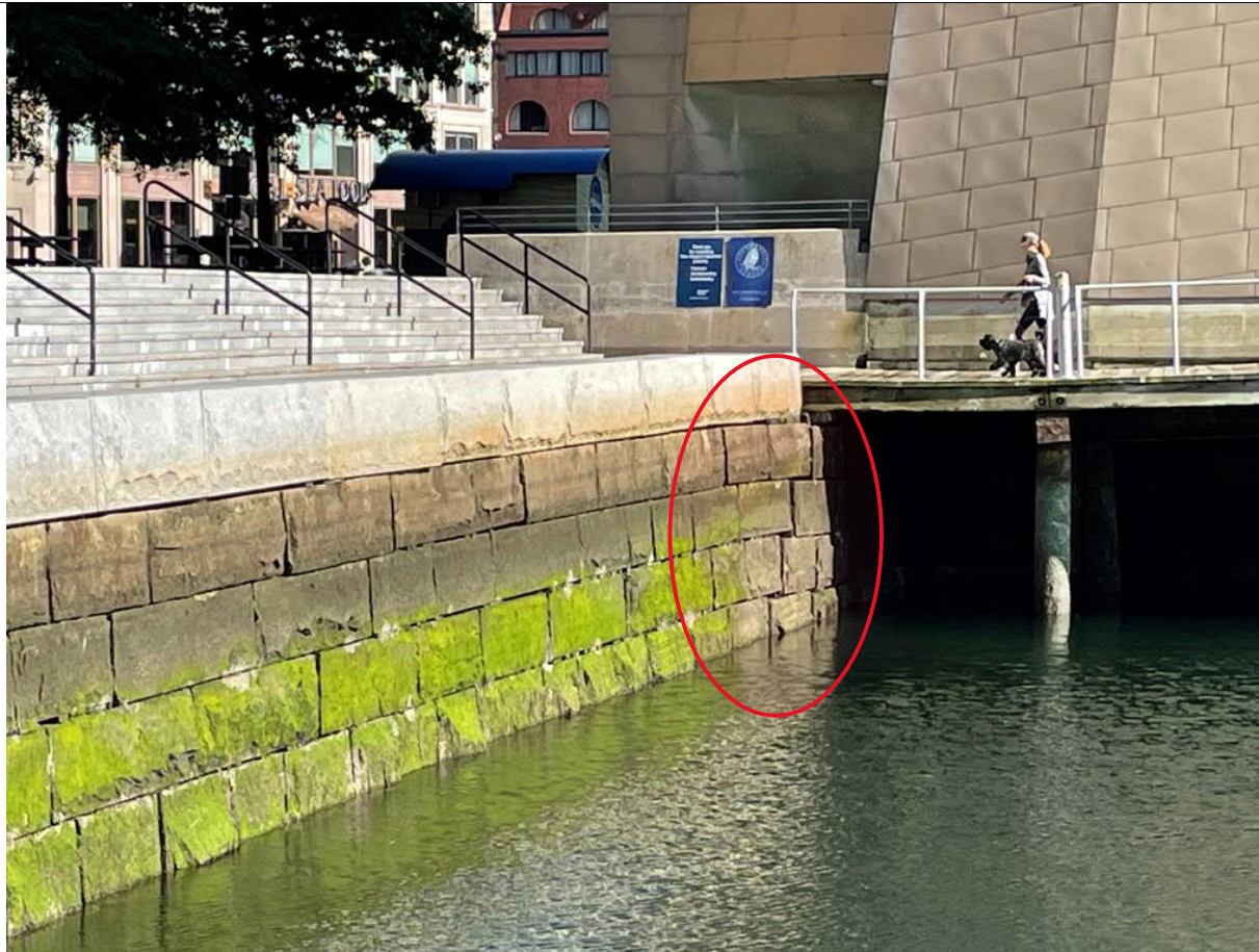
A – View of seawall, bearing failure at far end visible
