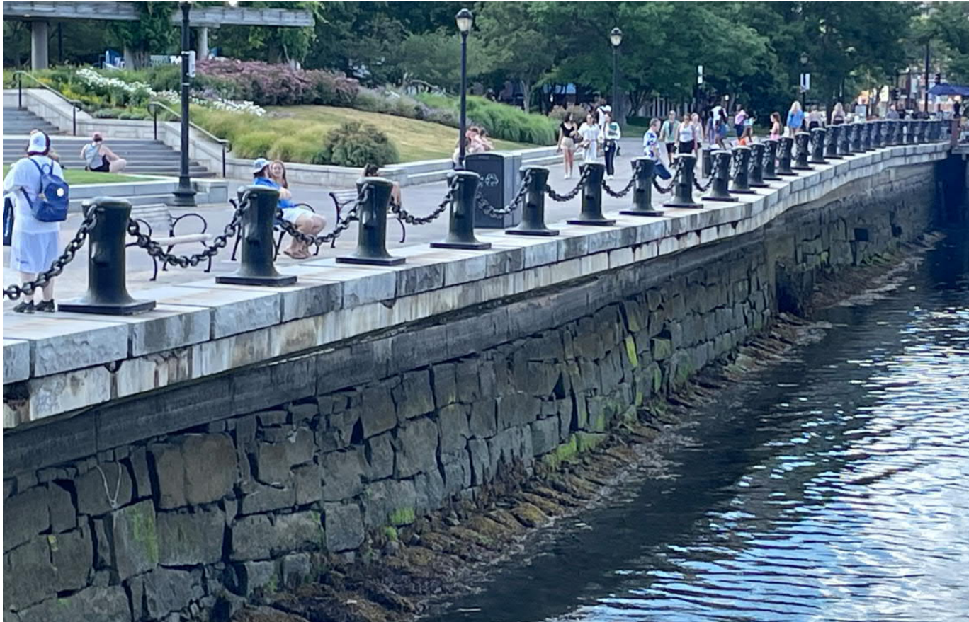
A – View of sea wall, note displacement of top of wall.
