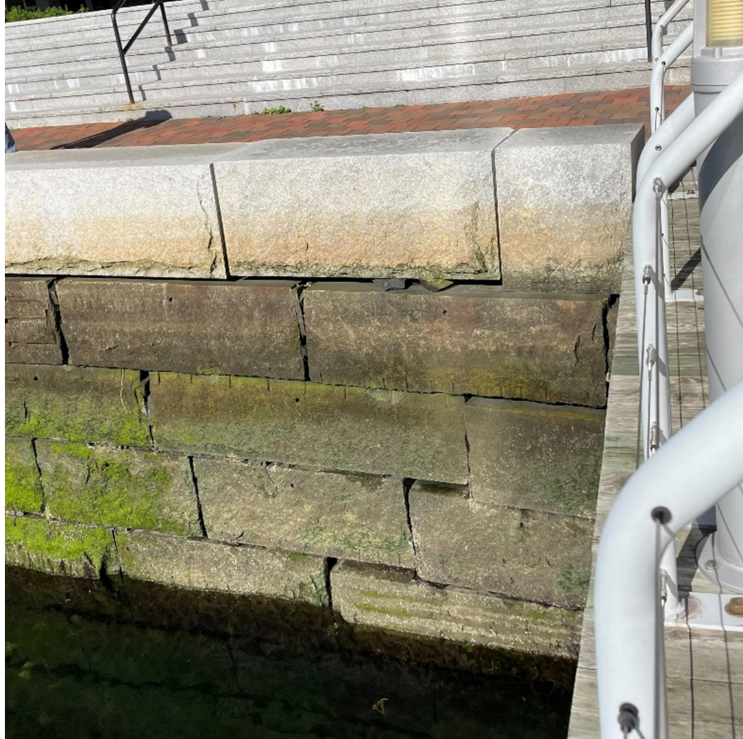
B – Detail showing crack/displacement at deck interface
