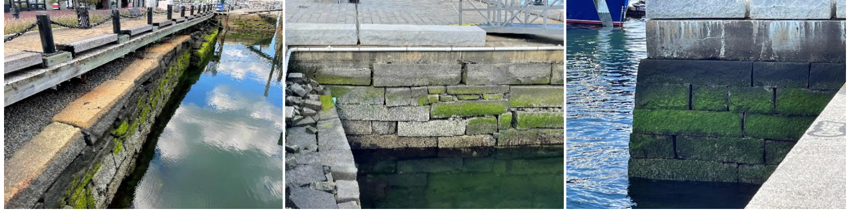
B – Typical South edge conditions – rebuilt granite seawall and existing granite seawall with concrete wall behind
