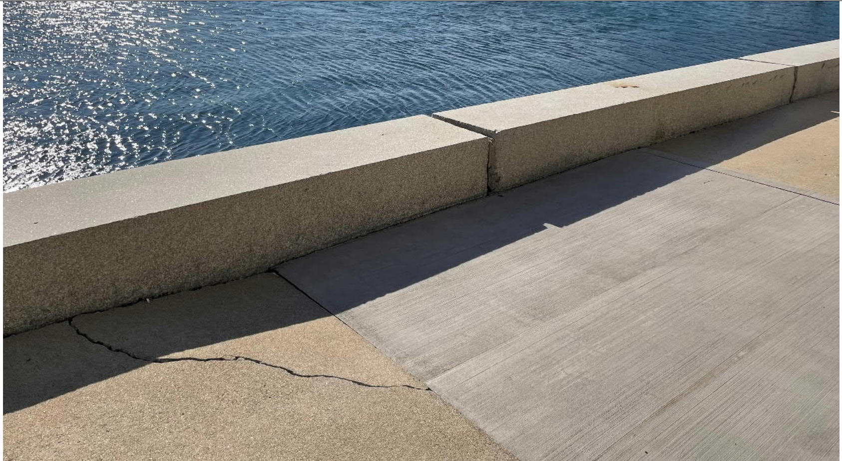
F – View of seawall (location 5) Settlement and cracking behind wall.
