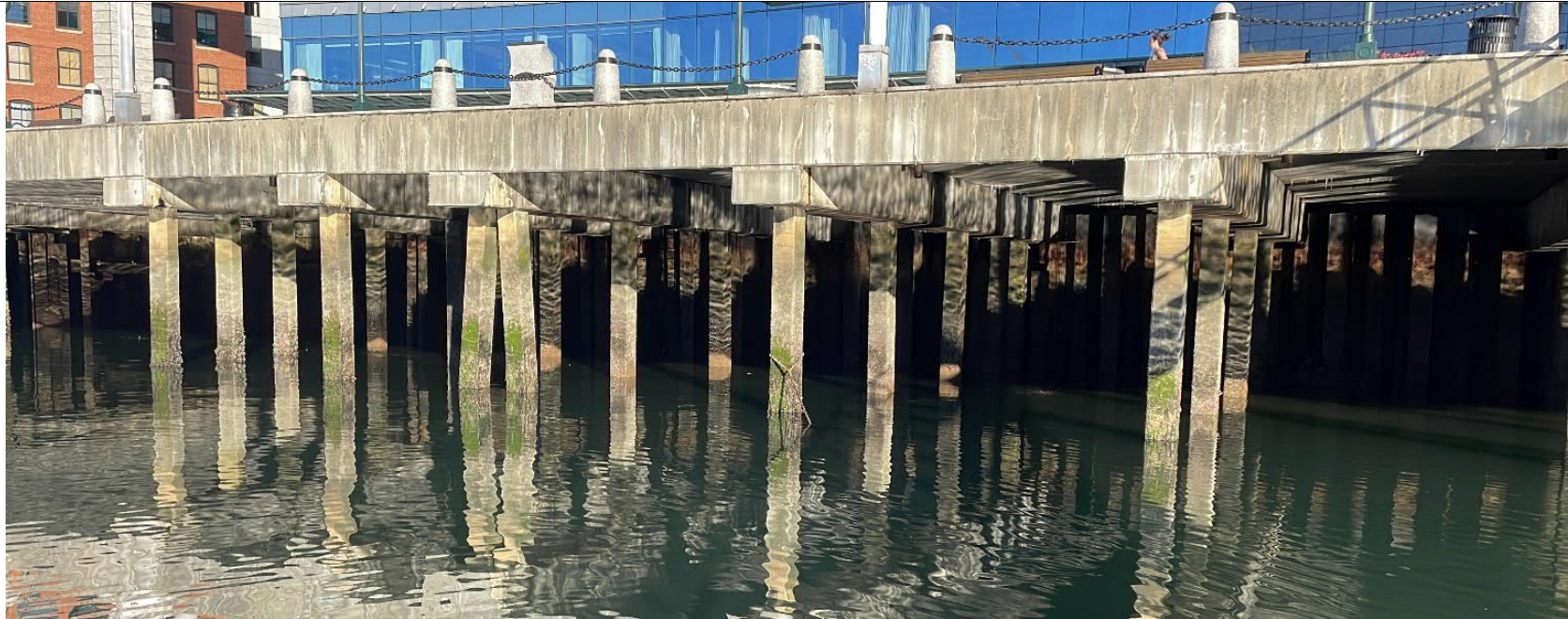
A – View of piers and deck with sheet pile sea wall visible in background
